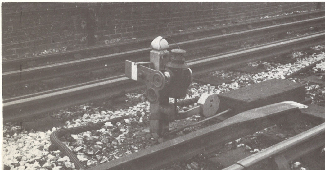
Bottom Semaphore shunt signal at Chesham station 15-4-67.
