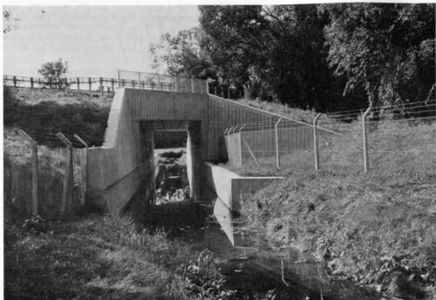
Above: View through the reconstructed bridge U24, looking south-west. [I. J. Robins
