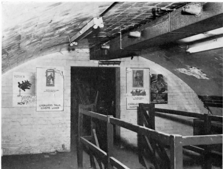
Above: The upper level of the King William Street station shelter. (By courtesy of David Ferris.)
