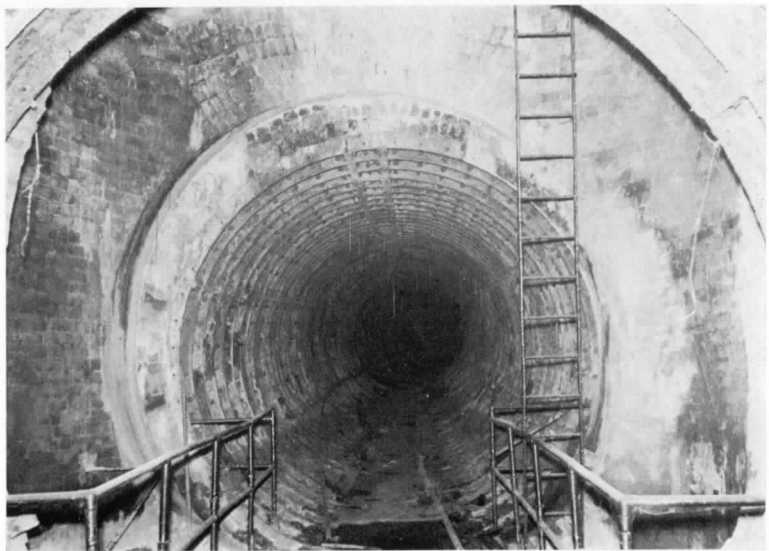
Below: Vertical construction shaft behind Old Swan Pier, at the lower tunnel level. The ladder goes up to the higher tunnel level. The drainage sump is below the walkway. (By courtesy of David Ferris.)
