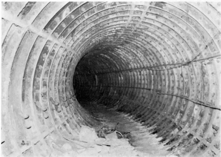
Below: 10ft 2ins internal diameter running tunnel, looking southwest under Arthur Street. (By courtesy of David Ferris.)
