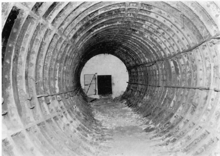
Above: One of the concrete plugs fitted with 4ft by 3ft watertight steel doors. The grill is an additional security measure. (By courtesy of David Ferris.)
