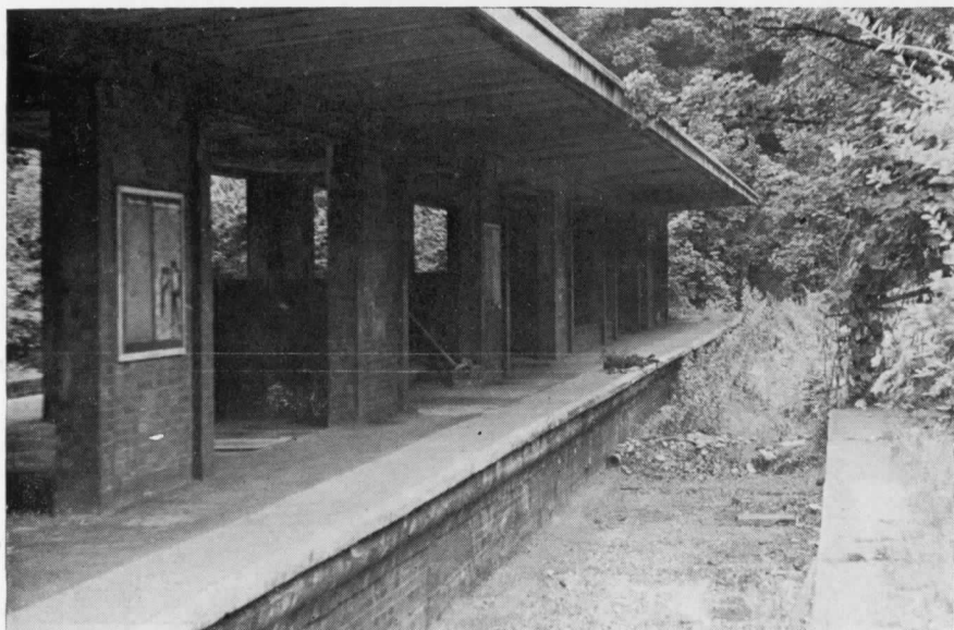
15. A view of Highgate high level station buildings a decade later, after occupation of the site by trees and undergrowth. Yet, a year later in 1980, all had been cleared because of drainage problems in the L.T. booking hall immediately underneath.
