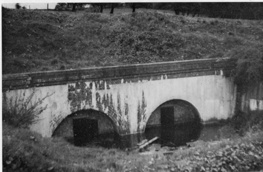
32. Work on the twin tube tunnels under Elstree Hill had commenced at the south end only, where the flooded bricked-up bores are seen in May 1958. These disappeared without trace in the mid-1960s during the construction of the M1 motorway, but not before a child was found drowned here in the 1950s. [Photomatic
