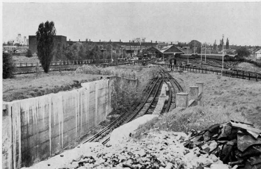
28. The same location almost a decade later, on 8th May 1965. The flyover bridge has been partly demolished, and the tracks leading to the Golders Green line (known as Nos. 17 and 18 sidings) were taken out of use in September 1964, and were removed shortly after this photograph was taken. The whole area is now overgrown and little can be seen of the 1939-40 works. [Alan A. Jackson]
