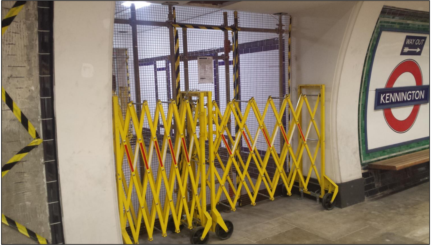
Above: New passageways built at Kennington have been unveiled but are not yet in use, as seen on 8 February 2020. The City branch platforms were closed between 26 May 2018 and 16 September 2018 during construction work.
