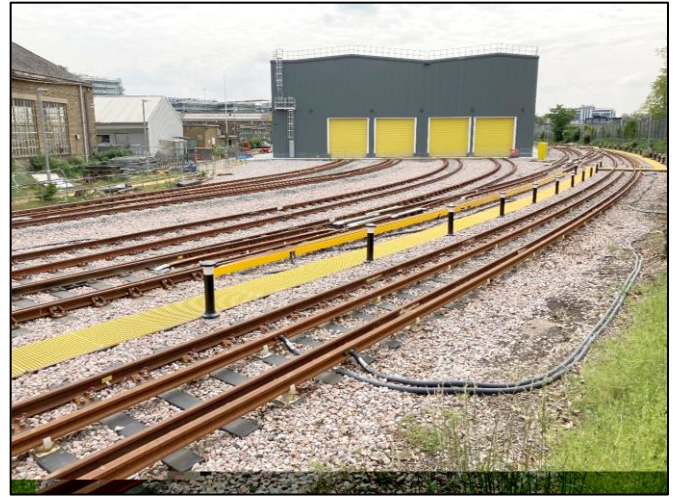
A major milestone was reached on 30 May 2021 at Acton Works where all ballasted track on roads 20, 21, 22, 23, 27 and 28 were handed over fit for the passage of trains.
