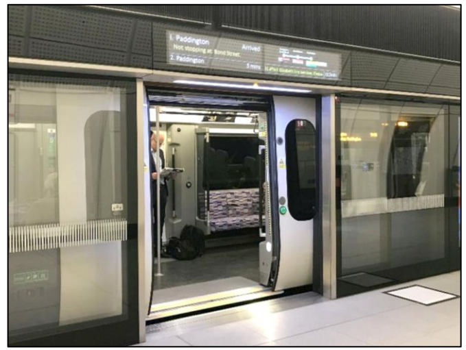
Platform Screen Door open with the Passenger Information Display above.
