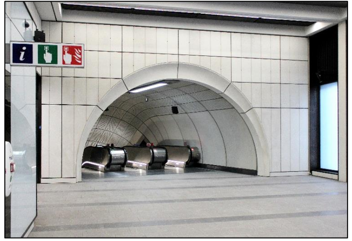
Above: The top landing of the 60m long escalators Nos. 13, 12 & 11 at Hanover Square.
