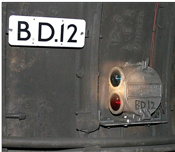
Figure 4: The current northbound inner home signal at Paddington Bakerloo. The case is the original AC supplied 'Style A' design used when the extension from Edgware Road was opened in 1913 and it is labelled McKenzie Holland and Westinghouse Power Signal Co. Ltd. This design was unique in having a circular case. Over the years, the signal has been renumbered and the position of the case may have changed. Photo: Tom Crane.
