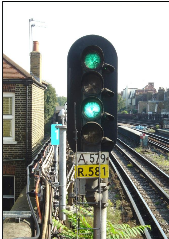
Figure 2: A comparison between a 4-aspect signal and a pair of two aspect signals on the same backplate. On the far left, JB3, the 4-aspect starting signal at Harrow-on-the-Hill Platform 1, shows a double yellow aspect, indicating two block sections ahead are clear. It also has an auxiliary red lamp below the main signal and a tripcock tester light to the left. On the left, two signals on a common backplate, at Stamford Brook (EB), both showing green. The upper green is for the stop signal while the lower one is for the repeater of the next signal. Photos by B. R. Hardy.
