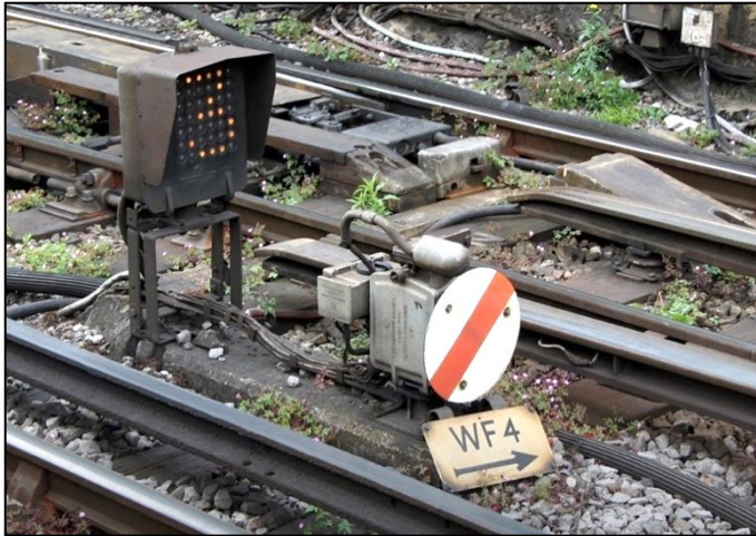
Figure 3: Standard Underground shunt signal with theatre type route indicator at Parsons Green (Code WF). The arrow on the signal plate points to the track that the signal affects. The signal rotates anticlockwise to show it is lowered. It is referred to as a lower quadrant shunt signal. The route indicator is showing '3', meaning it is set for the third route from the left. Photo: Kim Rennie.
