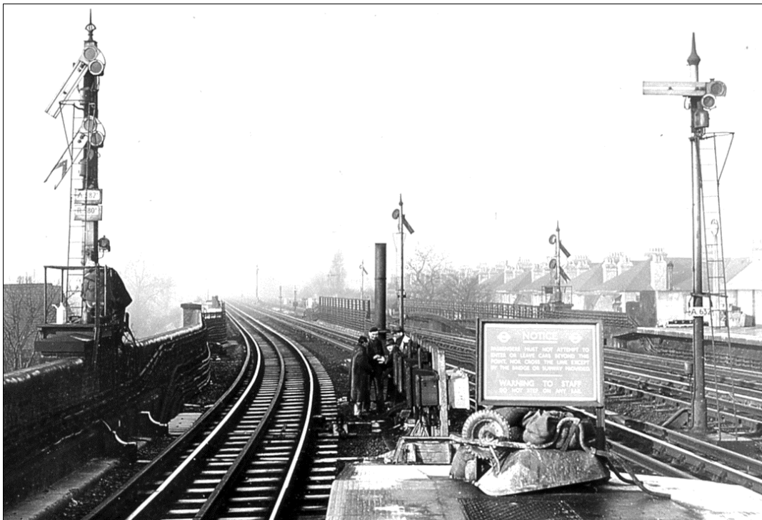
Figure 1 (left): A range of automatic electro-pneumatic semaphore signals as seen looking west from the westbound platforms at Stamford Brook. Many of them were installed for the four-tracking between Hammersmith and Acton Town, completed in 1932. The signals were replaced by colour lights in April 1952. Photo: LURS collection.
