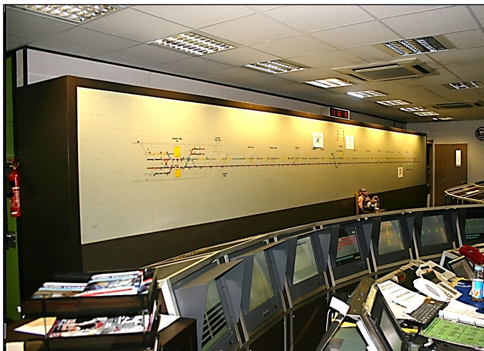
Figure 3: The interior of the Bakerloo room at the Baker Street SCC in November 2009. The whole line from Queen's Park (nearest the camera) to Elephant is shown. The VDUs are arranged at the desk provided with keyboard and mouse controls. Photo: Andrew Gardiner 2 .
