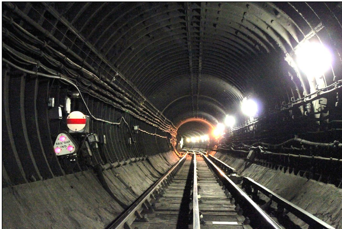
Figure 1: A superb photo of an illuminated Rail Gap Indicator at Hyde Park Corner. It is next to a standard disc type shunt signal. The RGI is illuminated because the traction current is switched off on the section ahead. The photo was taken during an inspection in non-traffic hours. Photo: Kim Rennie.
