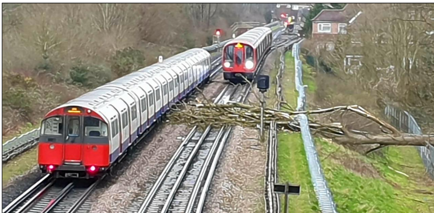
Above: The offending tree west of Rayners Lane, as viewed from Canon Lane road bridge and looking east towards Rayners Lane.
