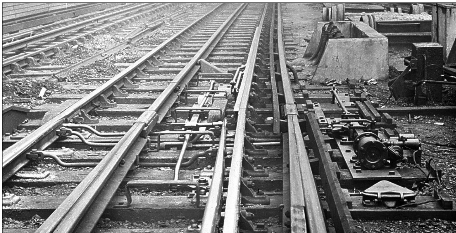
Figure 8: A set of District Railway facing points in 1905 with the pneumatic drive supplied by Westinghouse on the right of the track. All the parts shown in the drawing above can be seen here. Note the iron straps fixed over the locking in the four-foot. These supported wooden boards fitted over the top of the locking to protect it from equipment that might drop from trains. Note also the current rails are cut away and fitted with wooden fillets to allow clearance for the stretcher bars. Photo: Courtesy Westinghouse Archive & Chippenham Museum.
