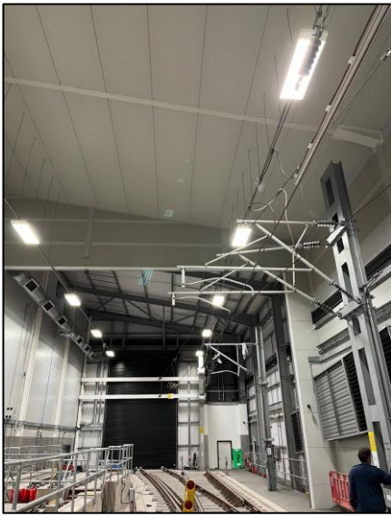
View of workshop looking east towards roller shutter door to outside track, showing overhead wiring.
