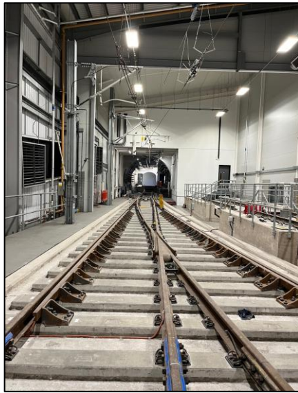
View of workshop with pointwork looking west back in towards the car mock-up in the distance.
